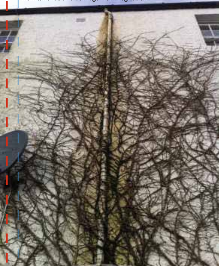
Inveraray, down pipe corroded and leaking through lack of maintenance and damage from vegetation
