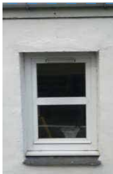
Window not in keeping with the character of the area
